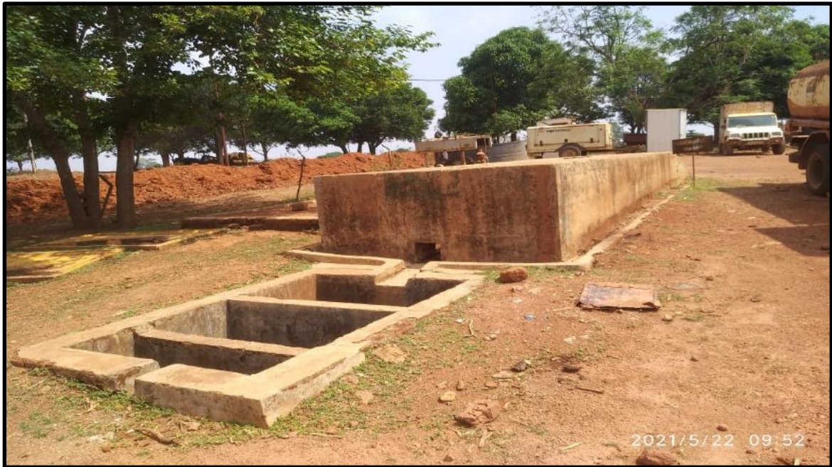
(Washing platform and oil & grease trap)
