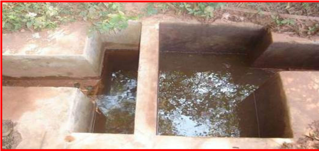
Oil & Grease separator
