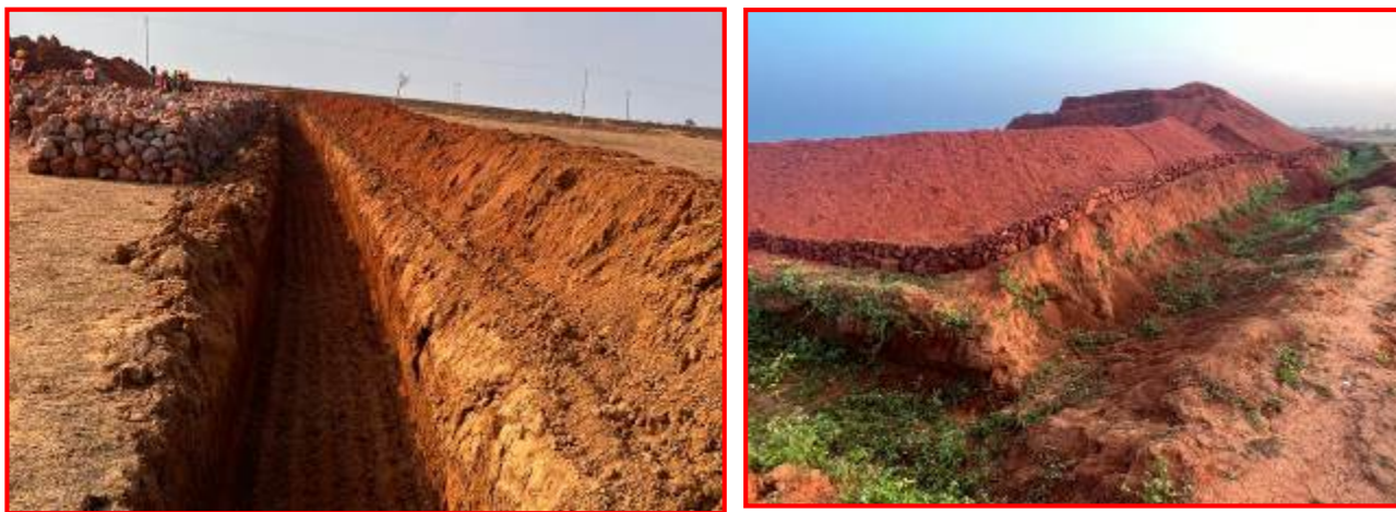
Garland drains around current Mine Pit
