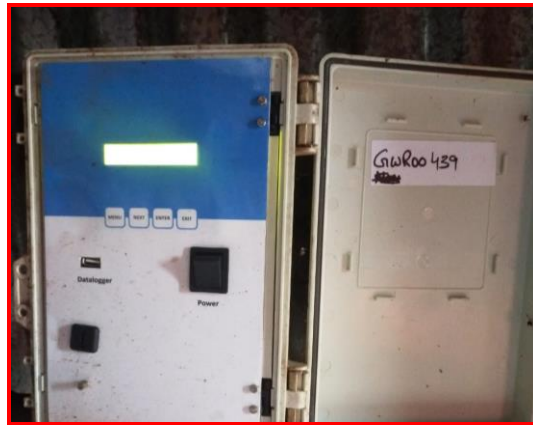
Piezometer at Kujam I Mine
