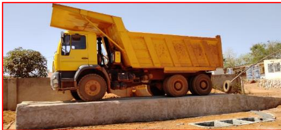
Washing ramp with Oil and Grease Trap
