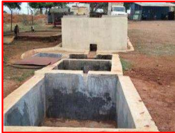
Washing Ramp and Oil and Grease Trap
