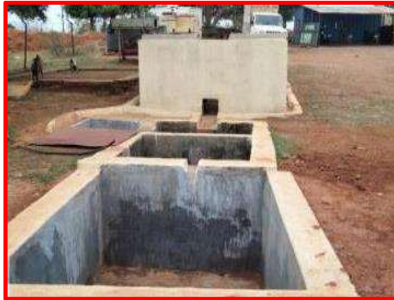
Washing Ramp and Oil and Grease Trap
