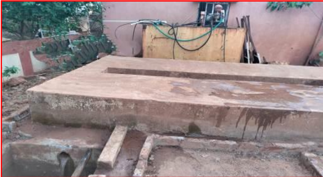
Washing Ramp with Oil and Grease trap
