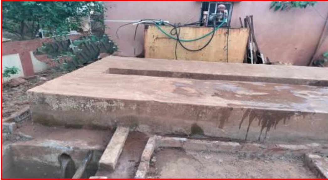
Washing Ramp with Oil and Grease trap
