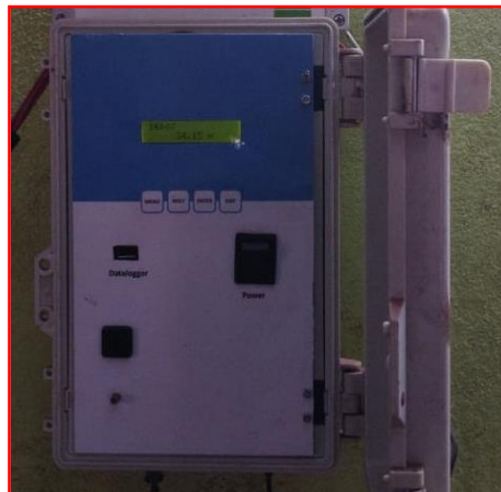
Piezometer Installed at Mine
