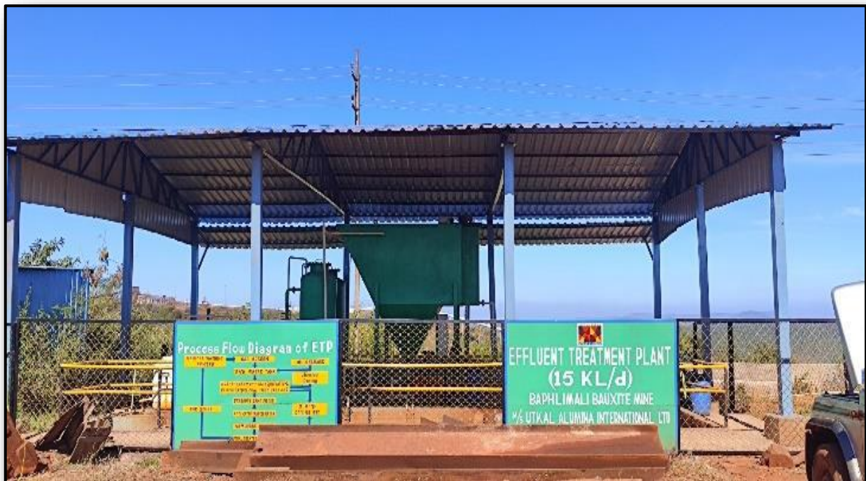
PHOTO 17: Showing 15 KLD Effluent Treatment Plant (ETP)
