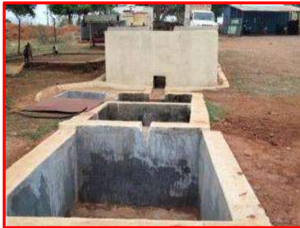
Washing Ramp and Oil and Grease Trap
