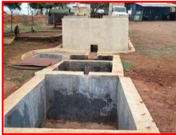
Washing Ramp and Oil and Grease Trap
