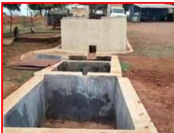
Washing Ramp and Oil and Grease Trap
