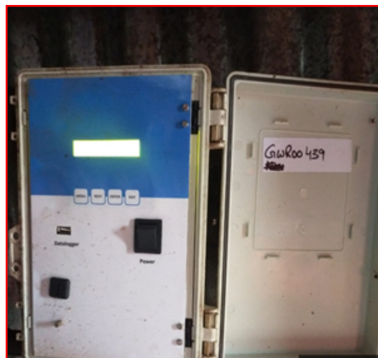
Piezometer installed at mine.
