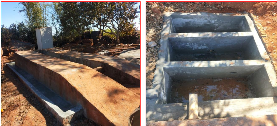
Oil and Grease Trap at Mines
