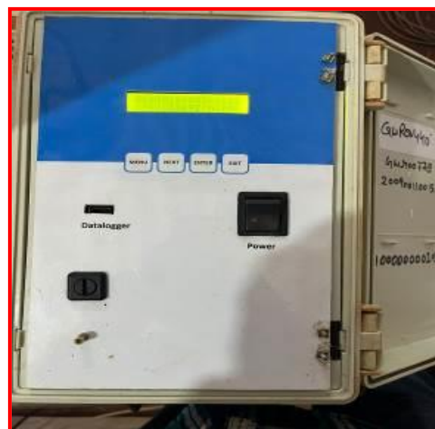
Piezometer Installed at Mine
