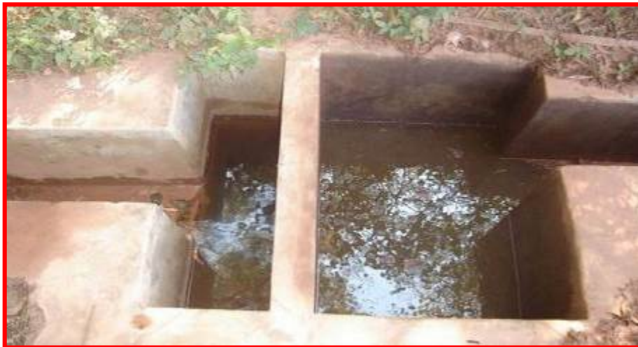
Oil & Grease separator
