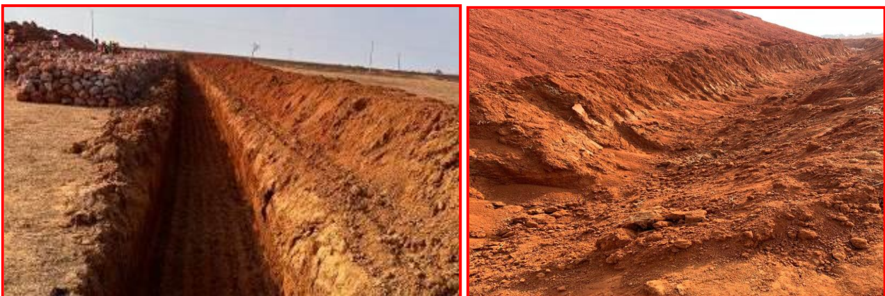
Garland drains around current Mine Pit
