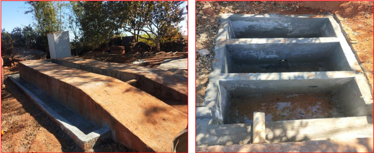
Oil and Grease Trap at Mines
