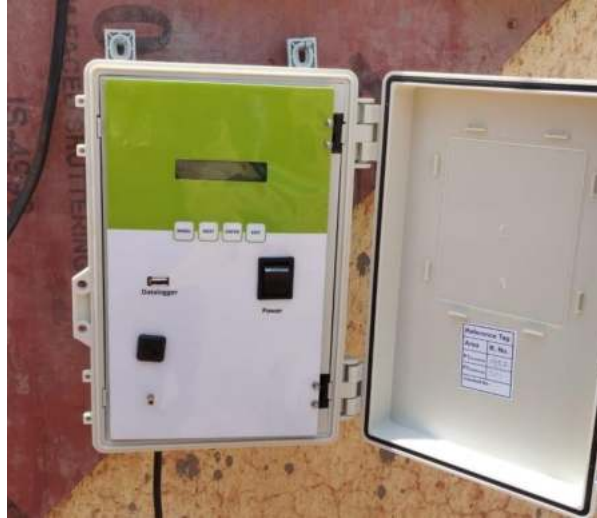
Piezometer at Amtipani Chirodih Mine
