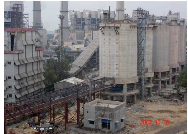
Ash Pipe rack to Silo
