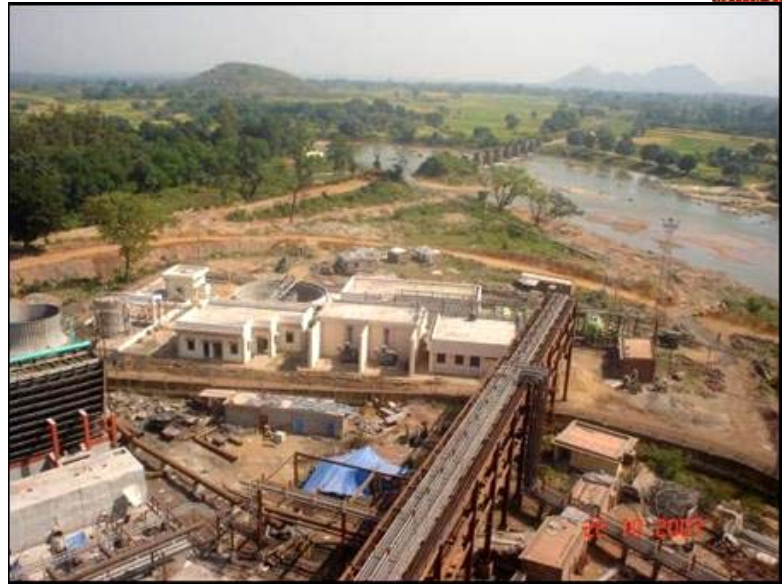
Raw water treatment & Effluent plant
