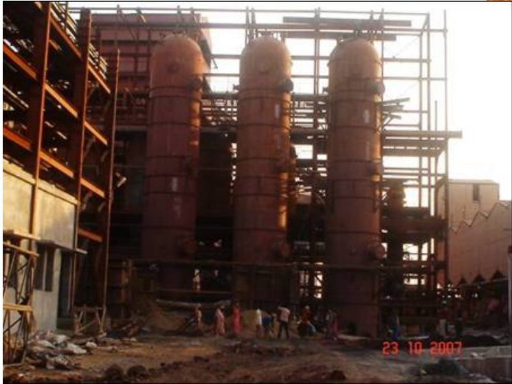
High Temp. Digesters
