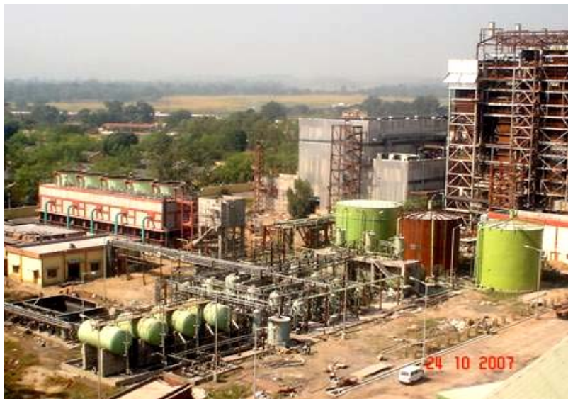
New Cogeneration Power plant view
