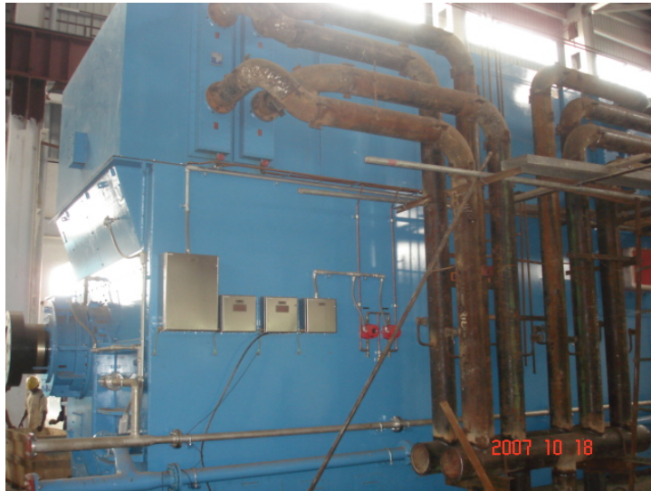
Generator on Foundation
