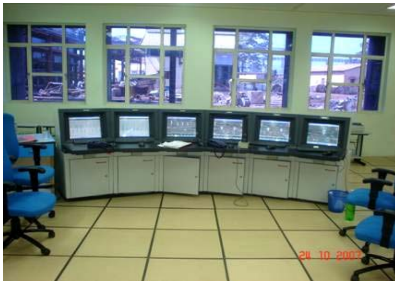
New Alumina plant DCS facility recently commissioned
