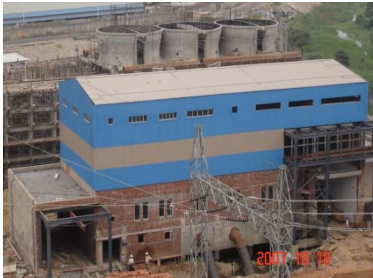
C W Pump House & Cooling Tower
