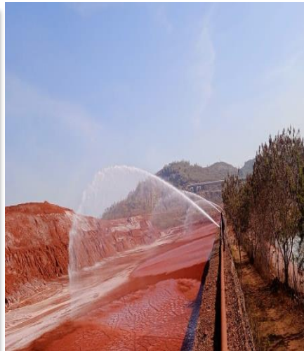
Fixed Sprinklers on RMDA
