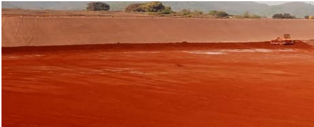
Slope correction for smooth water flow in monsoon at RMP B of Utkal
